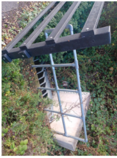
1. Broomhouse Lane, Edlington Trash Screen Checked before any predicted heavy rainfall events to assess requirement for cleansing.
