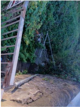
1. Sheffield Road, Conisbrough Trash Screen Checked before any predicted heavy rainfall events to assess requirement for cleansing.
